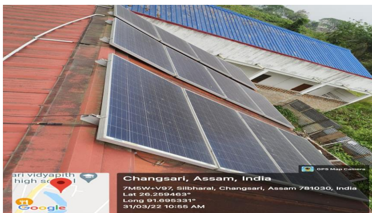
Photograph shows the roof-top solar panels in the college
